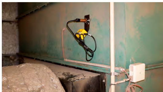
One of the sensors installed at the Tolefors drying plant.
